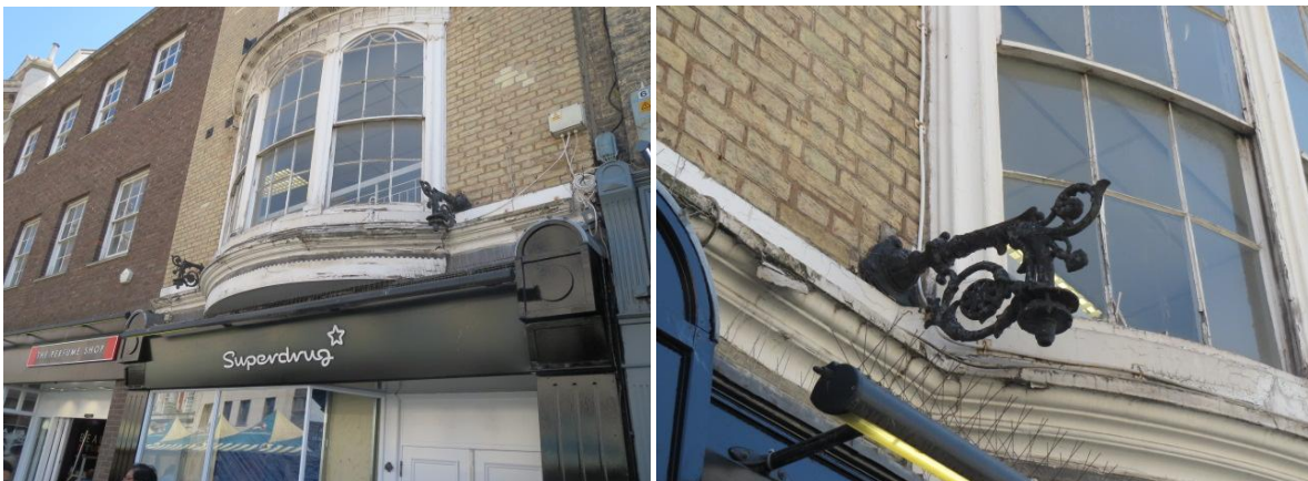
This bay window is in a sad state of repair currently.
